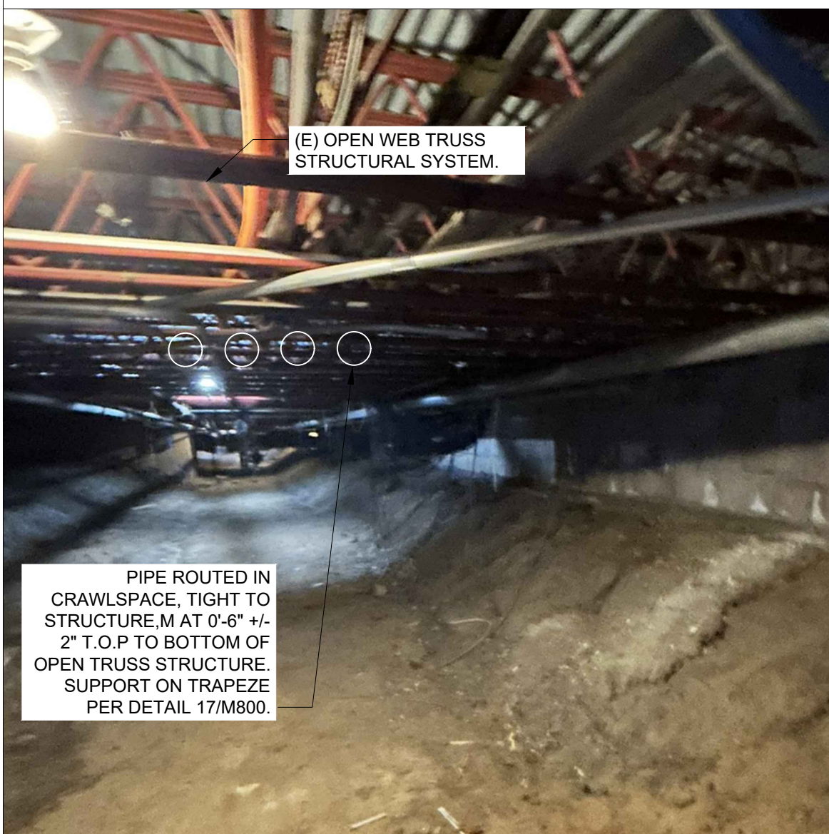
CRAWLSPACE PIPE ROUTING
