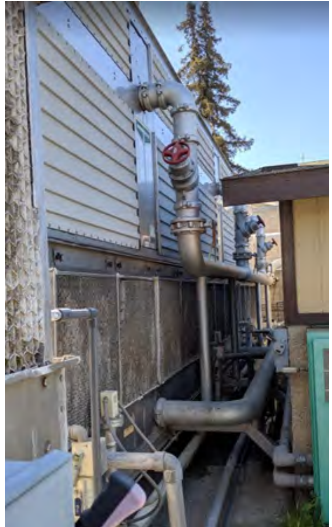
COOLING TOWERS FRONT AND BACK
