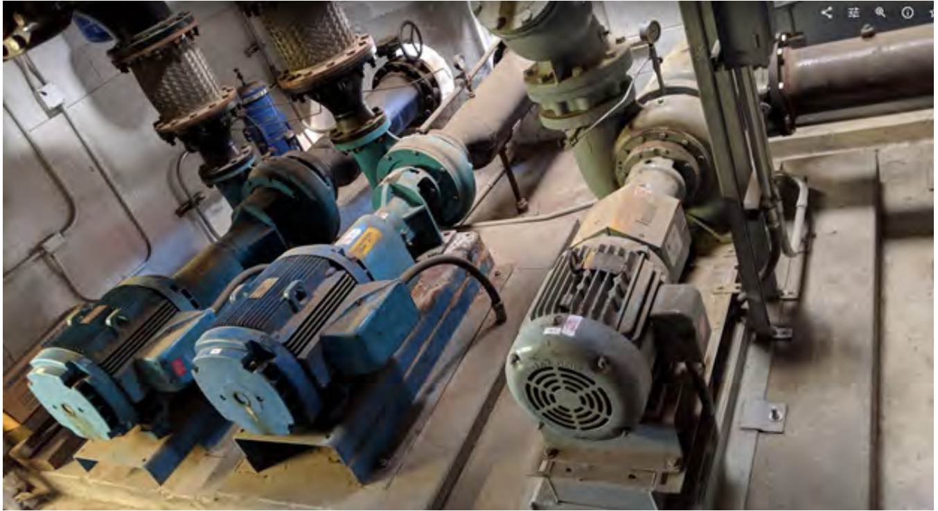
CONDENSER WATER PUMPS
