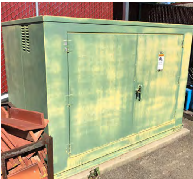
MID 21KV UTILITY SWITCH
