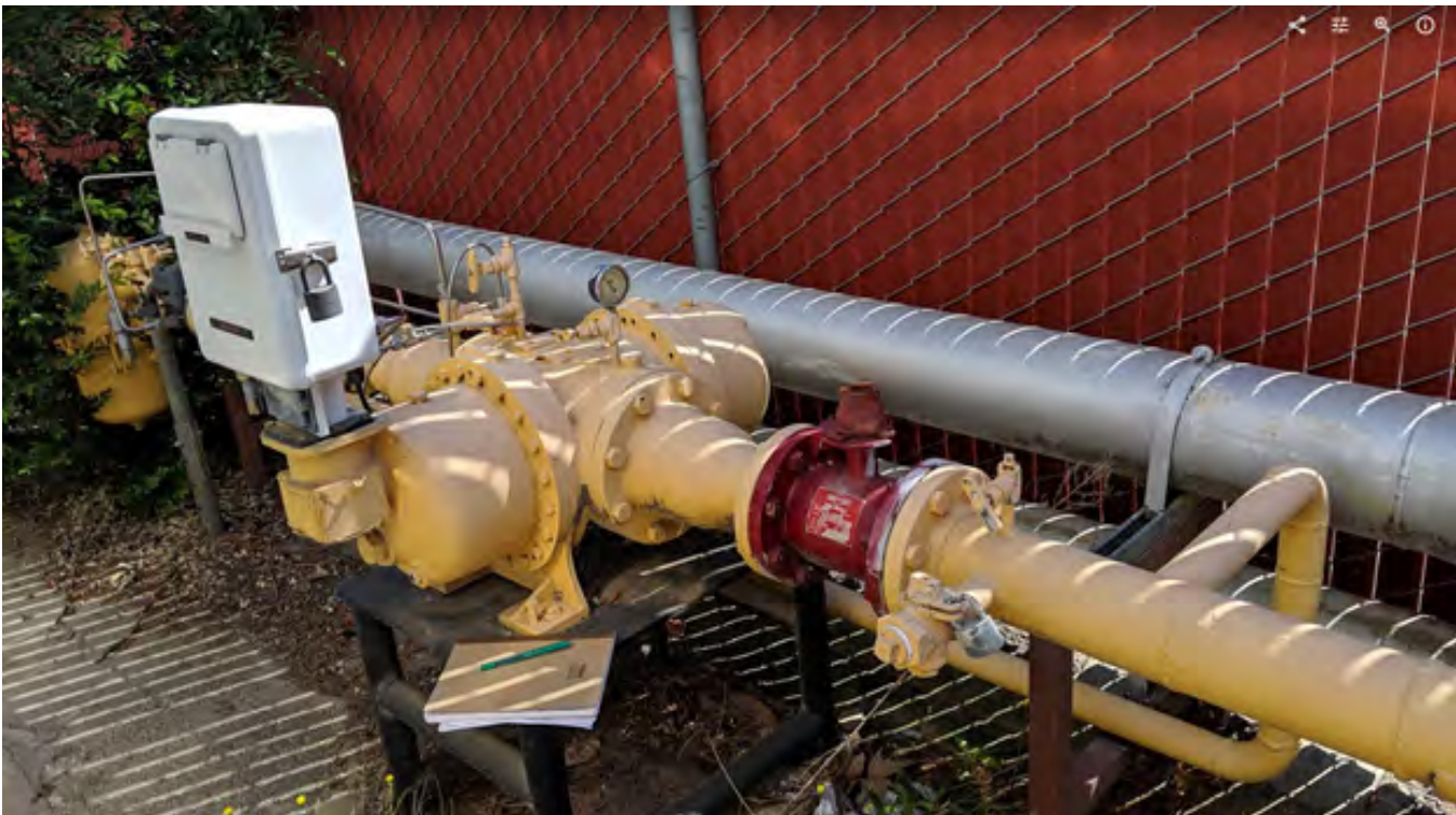
GAS METER AT CENTRAL PLANT
