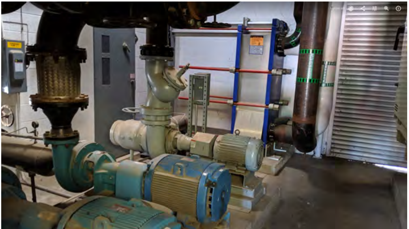
CONDENSER WATER PUMPS AND HEAT EXCHANGER FOR WATER-ECONOMIZER
