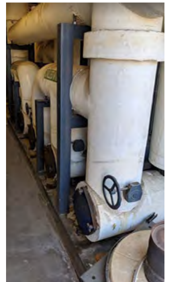
CHILLED WATER PUMPS 1 THROUGH 6
