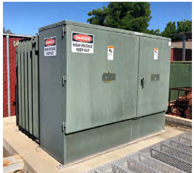
MID 21KV:12KV UTILITY TRANSFORMER
