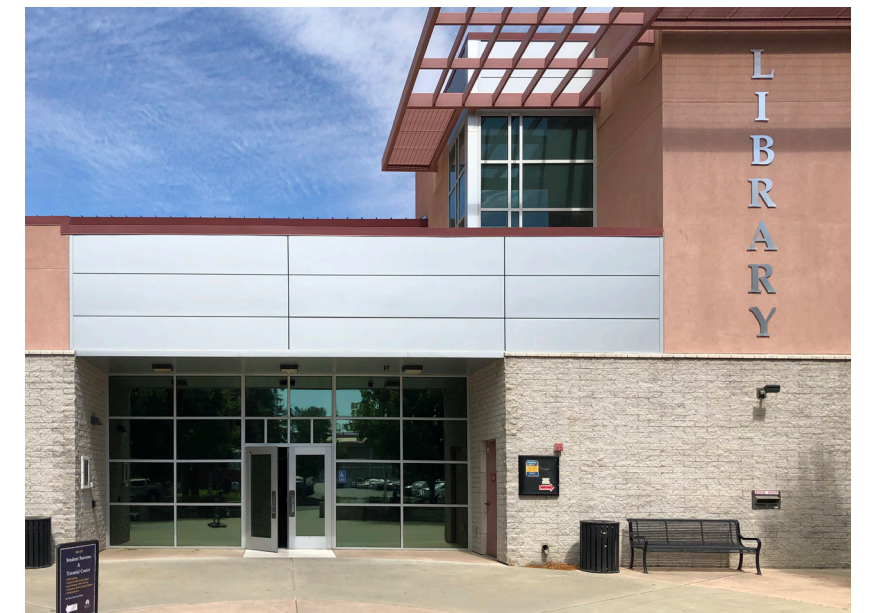
BROKEN FRONT DOOR OF THE LRC
